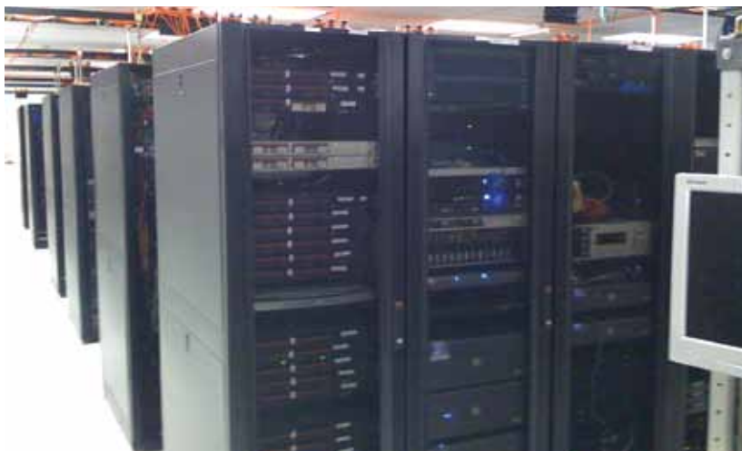
Computer servers connected to the internet.
